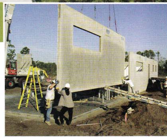
Lake Nona Fire Station 15 (above) was completed in September and sports a brightly painted green roof to complement its lush landscaping and other "green" specifications, like pre-cast "tilt" concrete walls (right).
